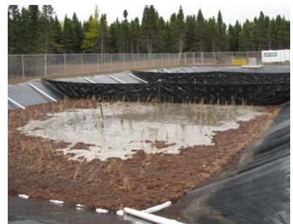
Sludge treatment cells
